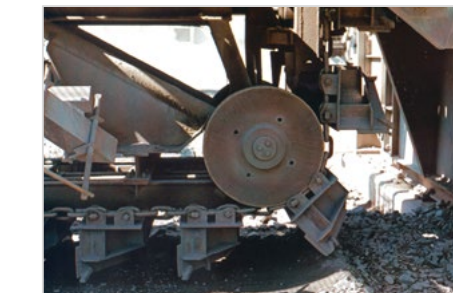
RECLAIMER SCRAPER BARS WITH SYSTEM 65
